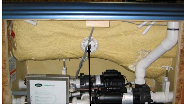
(Figure U) Light Bulb Location
