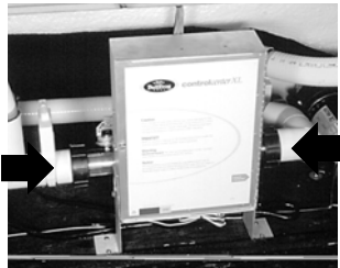
(Figure G) Spa Fittings
